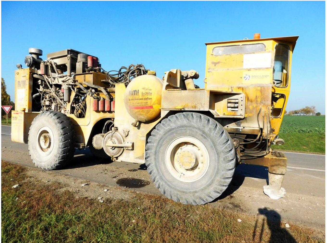
RB 500 resonance breaker – construction machine for demolishing the concrete substructure. Image: PORR AG
