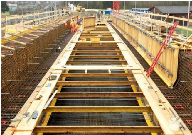
900m 3 of construction concrete was required for the construction of one section of the rail bridge. Image: PORR AG
