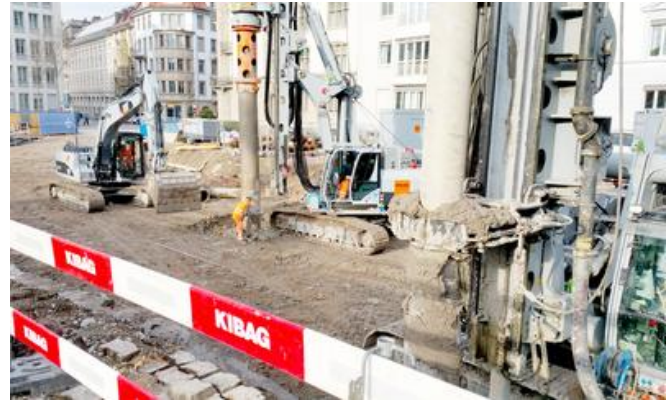
Foundation works to a depth of 17m: because of the construction site's location in the area of non-load-bearing lake deposits, the client decided against comprehensive refurbishment and in favour of a complete replacement of the building. Image: PORR AG
