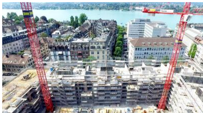
PORR employed a mixture of traditional load-bearing outer wall construction techniques for the upper floors. Image: PORR AG
