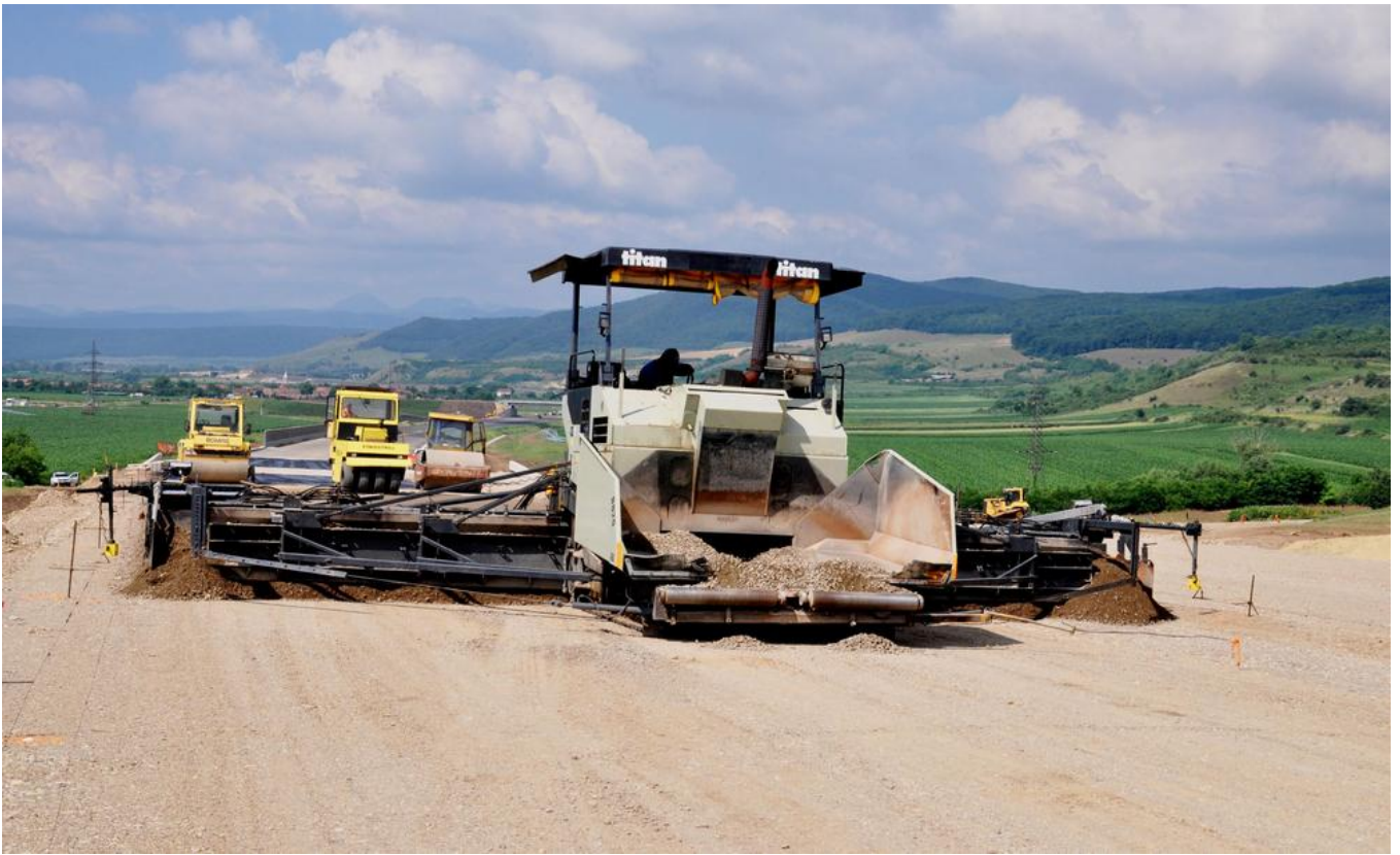
Installation of the hydraulically-bound base course with a finisher. Image: PORR AG
