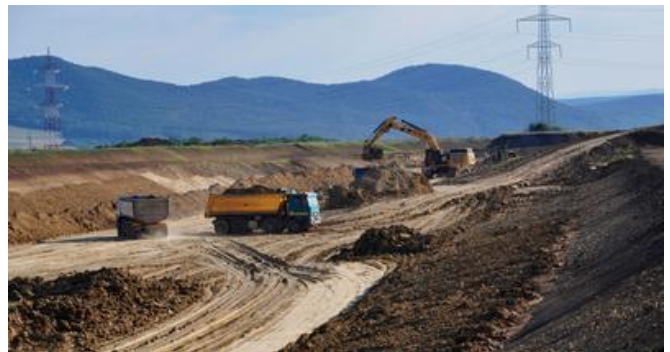
A 220kV power mast right in the middle of the motorway had to be relocated. Image: PORR AG
