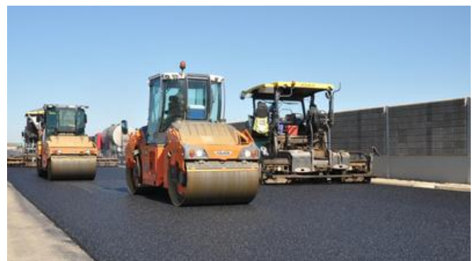
Working on high pressure: Asphalt works on the new motorway. Image: PORR AG
