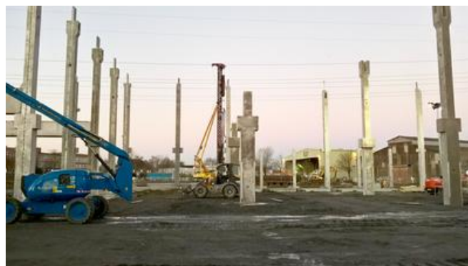
From October 2016, the foundation works were running in parallel with construction of the structural carcass. Image: PORR
