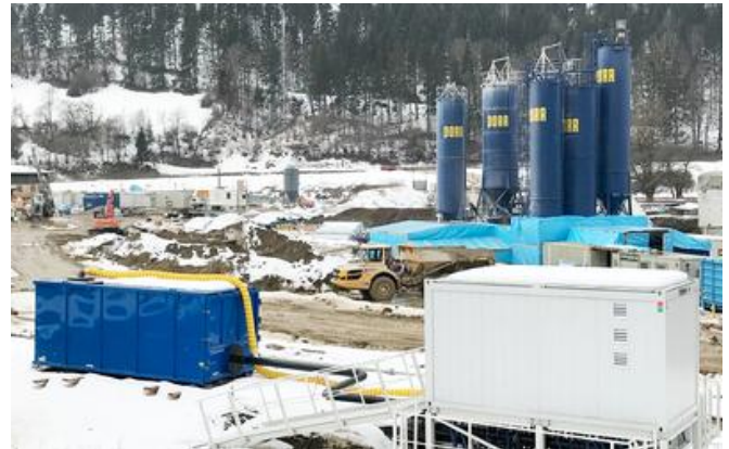
Soil gas extraction system (blue container) with a temporary exhaust line during ongoing site work. Image: PORR Umwelttechnik GmbH
