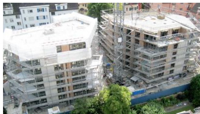
Generous wood-aluminium windows are part of the high-quality façade. Image: PORR AG
