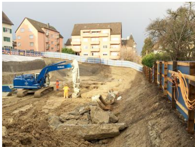
The construction pit following demolition of the largest New Apostolic Church in Switzerland. Image: PORR AG
