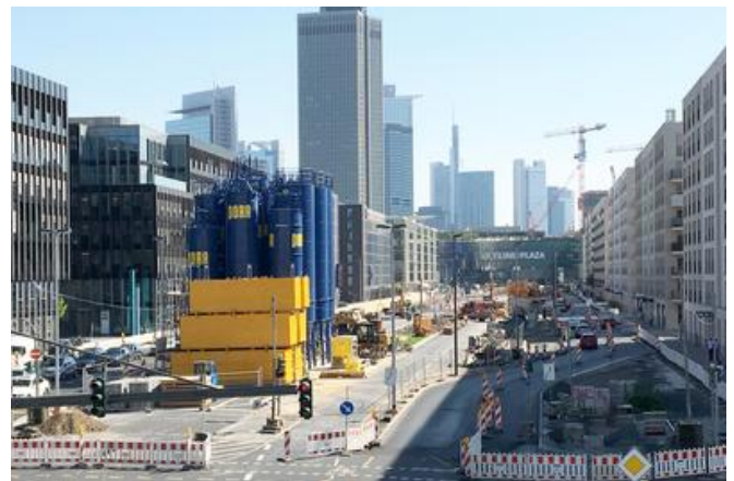
Site facilities and traffic lane reduction on the Europa Allee. Image: PORR AG
