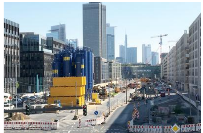
Site facilities and traffic lane reduction on the Europa Allee. Image: PORR AG
