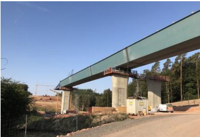
Six weeks of metalwork and welding preceded the successful launch. Source: PORR
