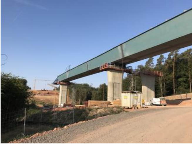
Six weeks of metalwork and welding preceded the successful launch. Source: PORR
