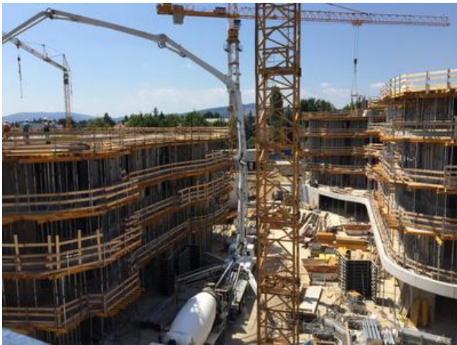
The formwork for the 3 km of balcony edge beams presented a particular challenge. Source: PORR
