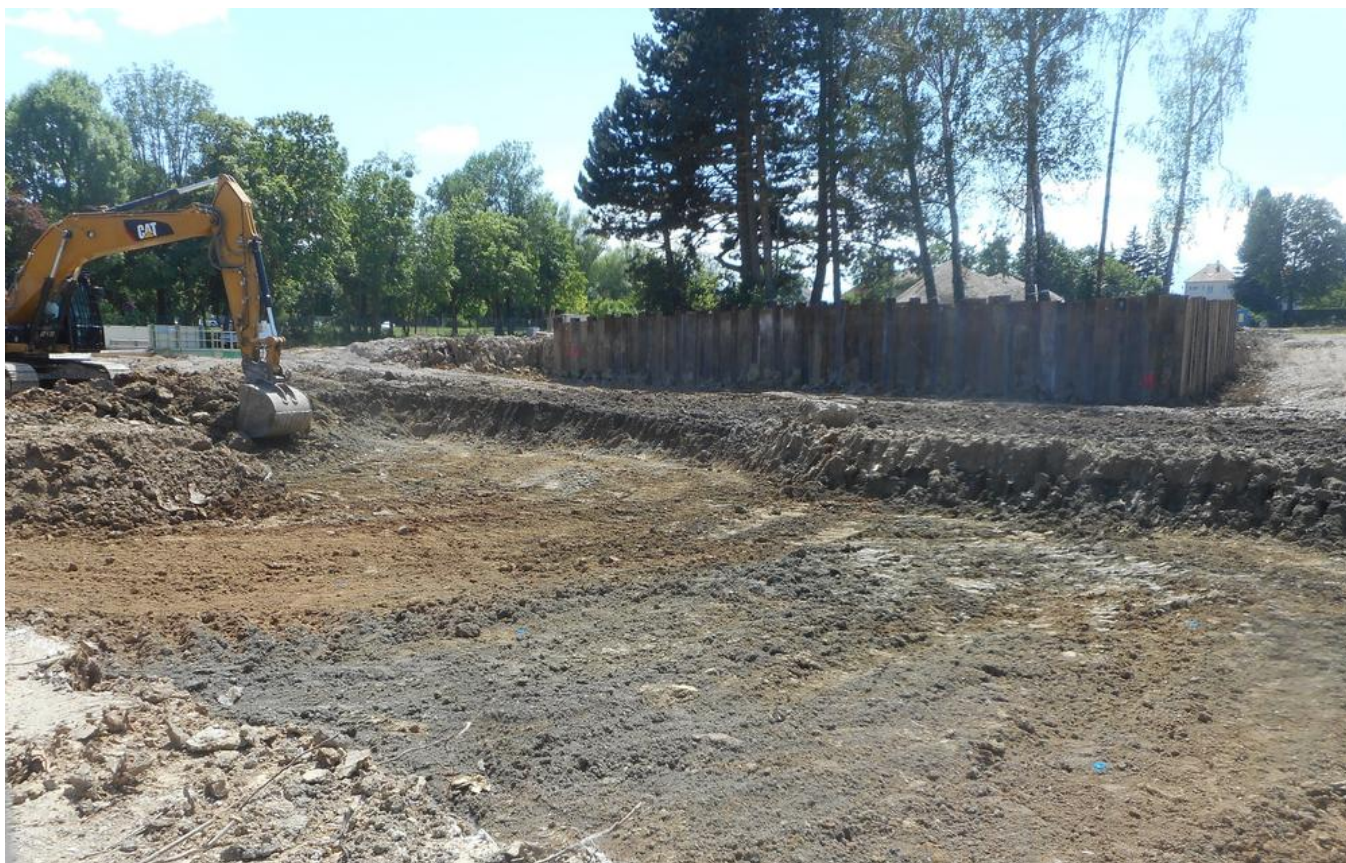
During the foundation work, a group of trees in the middle of the construction site had to be taken into account... Source: PORR
