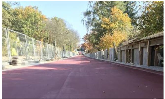
Caption: A new road surface was applied on the bridge and its ageing concrete rails were replaced. Source: PORR
