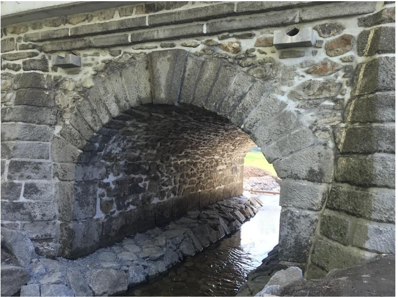
The visible areas of jointing were neither smoothed nor treated in any other way. Missing parts of the natural stone masonry were filled in using rubble. Source: PORR
