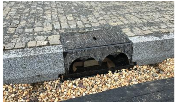
Caption: Even the kerb drainage systems needed to correspond to the specifications set down by the Monument Care Department. Source: PORR
