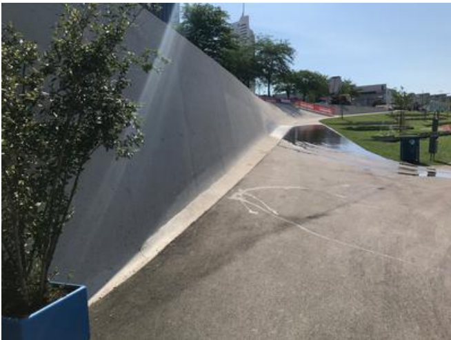
Custom-made formwork was needed to produce the exposed concrete surfaces. Source: PORR
