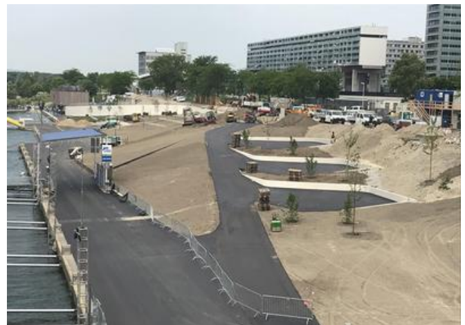
PORR erected several retaining walls featuring irregular curves along the embankment area. The largest retaining wall begins at the quay and ends at the top of the embankment (visible in the background). Source: PORR
