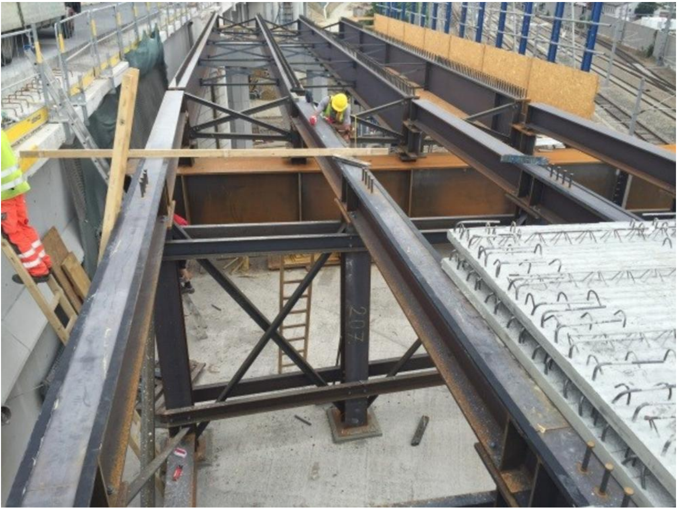
To create space for the construction site facilities and maintain ongoing traffic, the lanes were temporarily widened with the aid of composite steel bridges. Source: PORR
