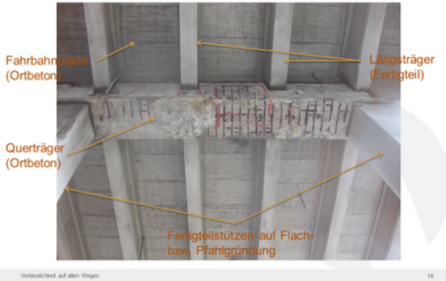
The steep increase in lorry traffic and prolonged use of road salt have resulted in irreparable damage. Source: PORR
