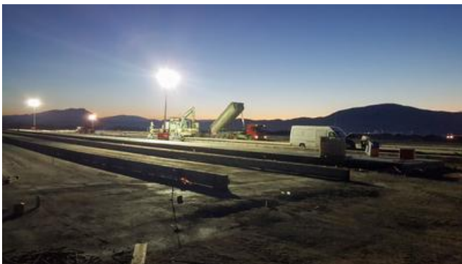
Solid steel girders were used as formwork for the concrete layer. Source: PORR Construct
