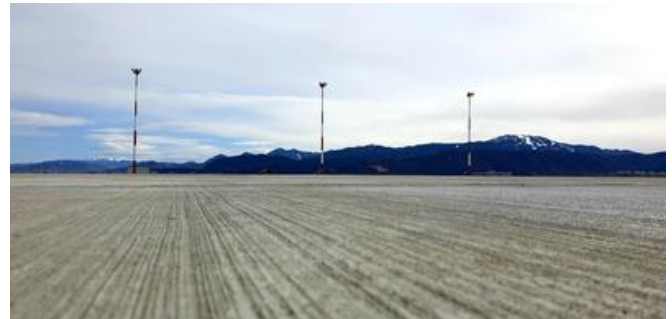
PORR built a high-mast lighting system at the edge of the platform. Source: PORR Construct
