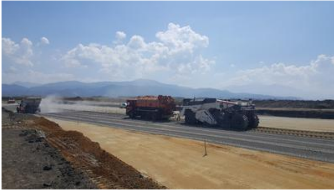
A 25cm thick stabilised ballast layer was laid on top of the lower ballast layer for the taxiway and apron. Source: PORR Construct
