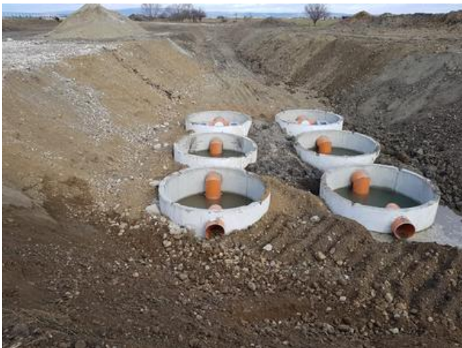
Water is cleaned in the two-stage oil separator system. Source: PORR Construct
