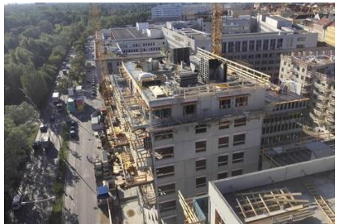
The overhanging balconies in the three top storeys presented a major challenge during the carcass construction. Source: PORR
