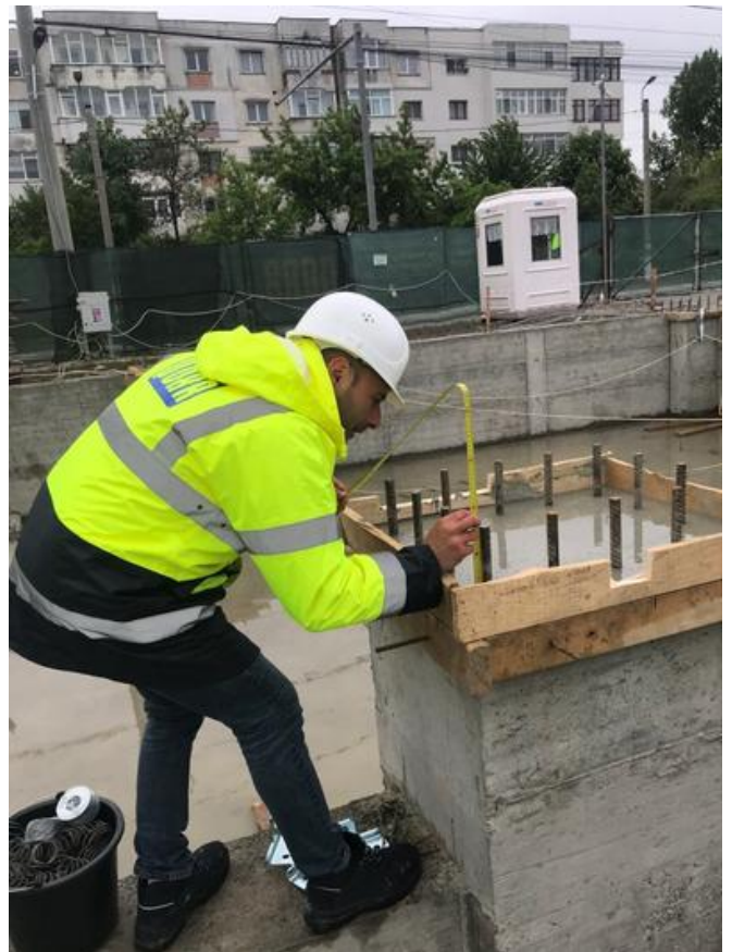
The rebars had to be placed with a maximum deviation of 5mm, in order that the grout sleeves could be assembled precisely on the prefabricated columns. Source: PORR Construct
