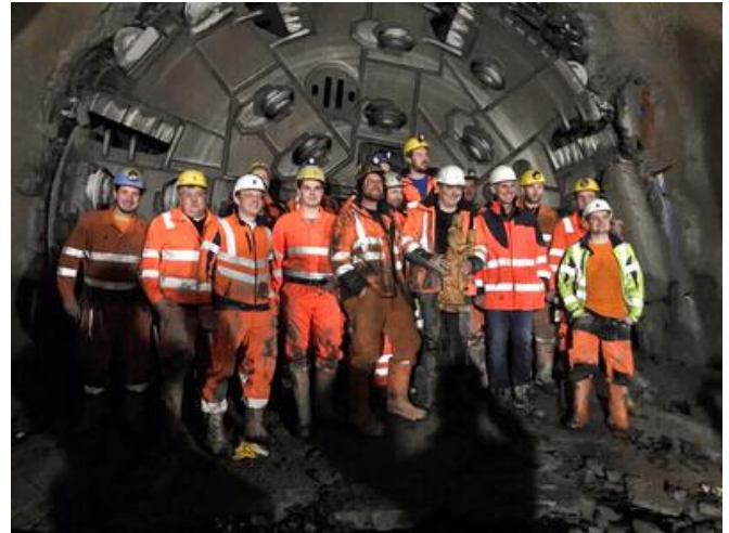
The northern section of the headrace tunnel was the first to be broken through, in April 2019. Source: GKI Maria Stein consortium
