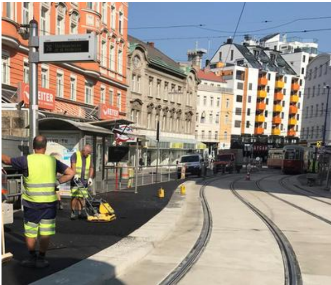
The final stage was to install asphalt between the guide wall element and the road at the tram stops. Source: PORR AG
