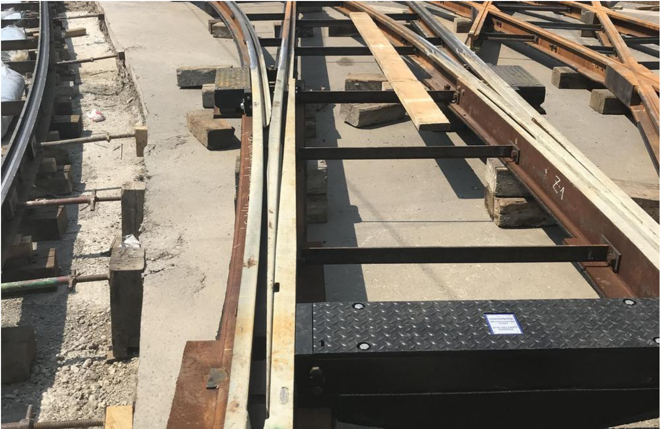
The grooved swivel plates for the intersection were pre-installed. Source: PORR AG
