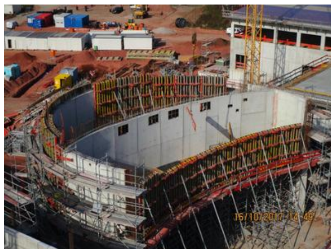
The stage tower has a curved reinforced concrete wall that was a significant challenge to build. Source: BBGS GmbH
