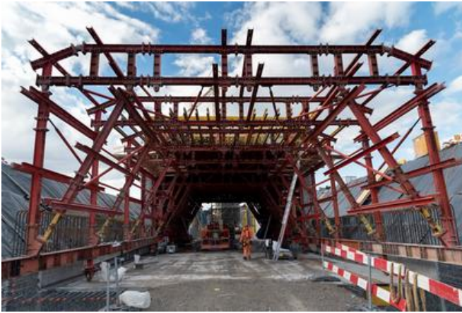
Formwork carriage and secondary carriage during assembly for use in the next 32 ceiling casting stages. Source: PORR
