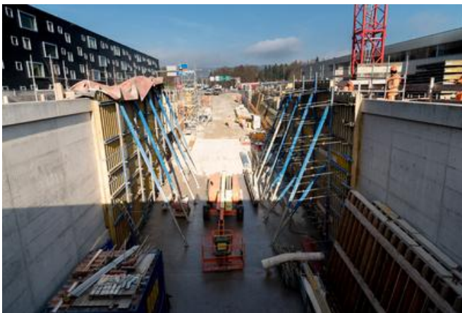
The Hero ramp during construction of the ramp walls in November 2019. Source: PORR
