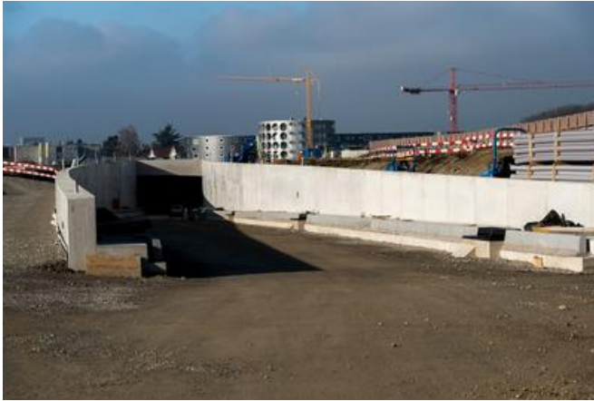
The completed Horner ramp with strip foundations and verge in place. Source: PORR
