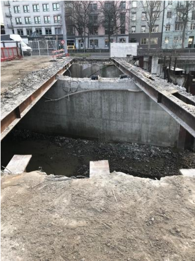
Around 380t of steel was removed when the old Postbrücke was dismantled. Source: PORR
