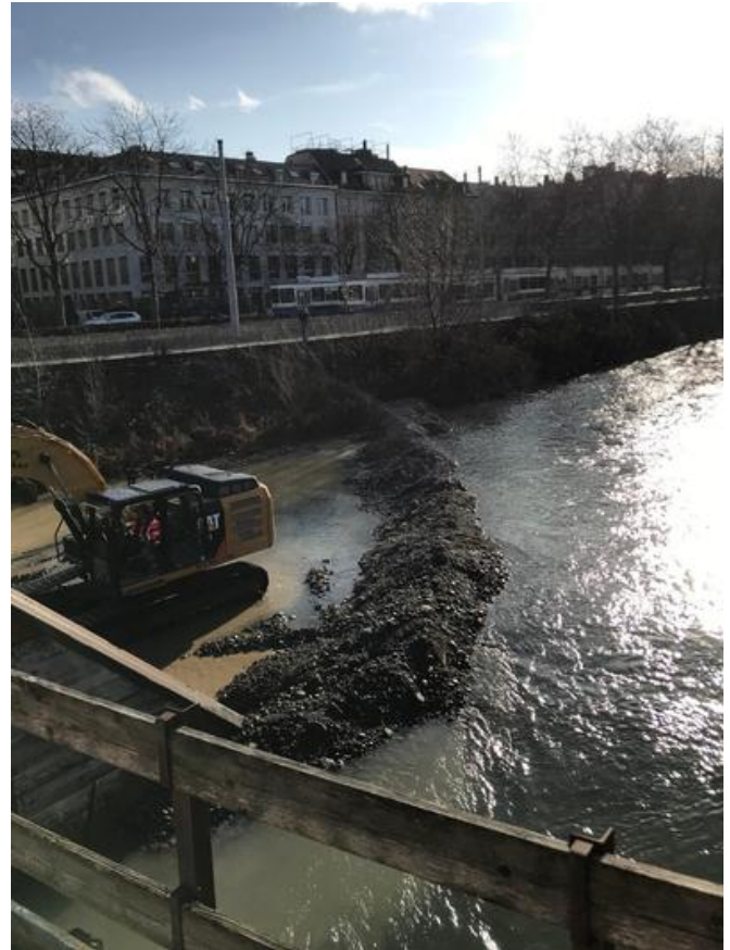
In order to allow the dismantling process to be carried out seamlessly, floodable embankments were created to expose the riverbed beneath individual spans. Source: PORR
