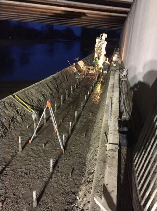
The small bored piles for the skidways were constructed by PORR Grundbau. Source: PORR
