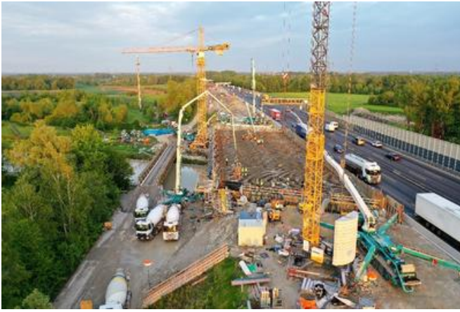
The delivery of concrete for concreting the superstructure proved to be a real challenge because of the high volume of traffic. Source: PORR
