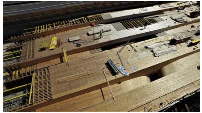
The load-bearing formwork was constructed with parabolic longitudinal girders and conical piers. Source: PORR
