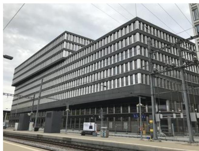
A large, cantilevered section was constructed above the first floor, with loads from the eight floors above applied to this section. Source: PORR
