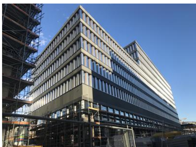
The building on site B was realised as a reinforced concrete skeleton construction. Source: PORR
