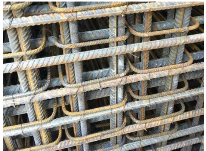
The complexity of the frame and the jointless construction resulted in a complicated reinforcement layout with very high reinforcement density of the individual components. Source: PORR
