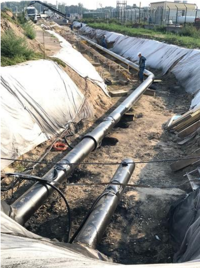
The damaged pipeline had to be excavated along a length of 140m in preparation for replacement. Source: PORR
