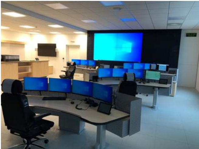
The operations control room is built on an earthquake-resistant raised floor. Source: PORR
