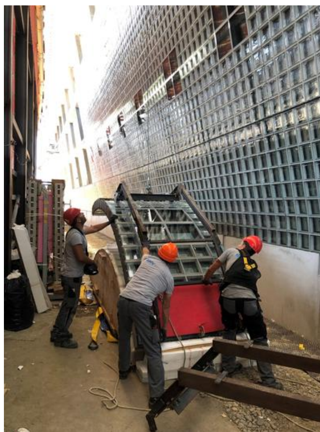
Hoisting the elements into place proved particularly challenging due to the cramped conditions. Source: PORR
