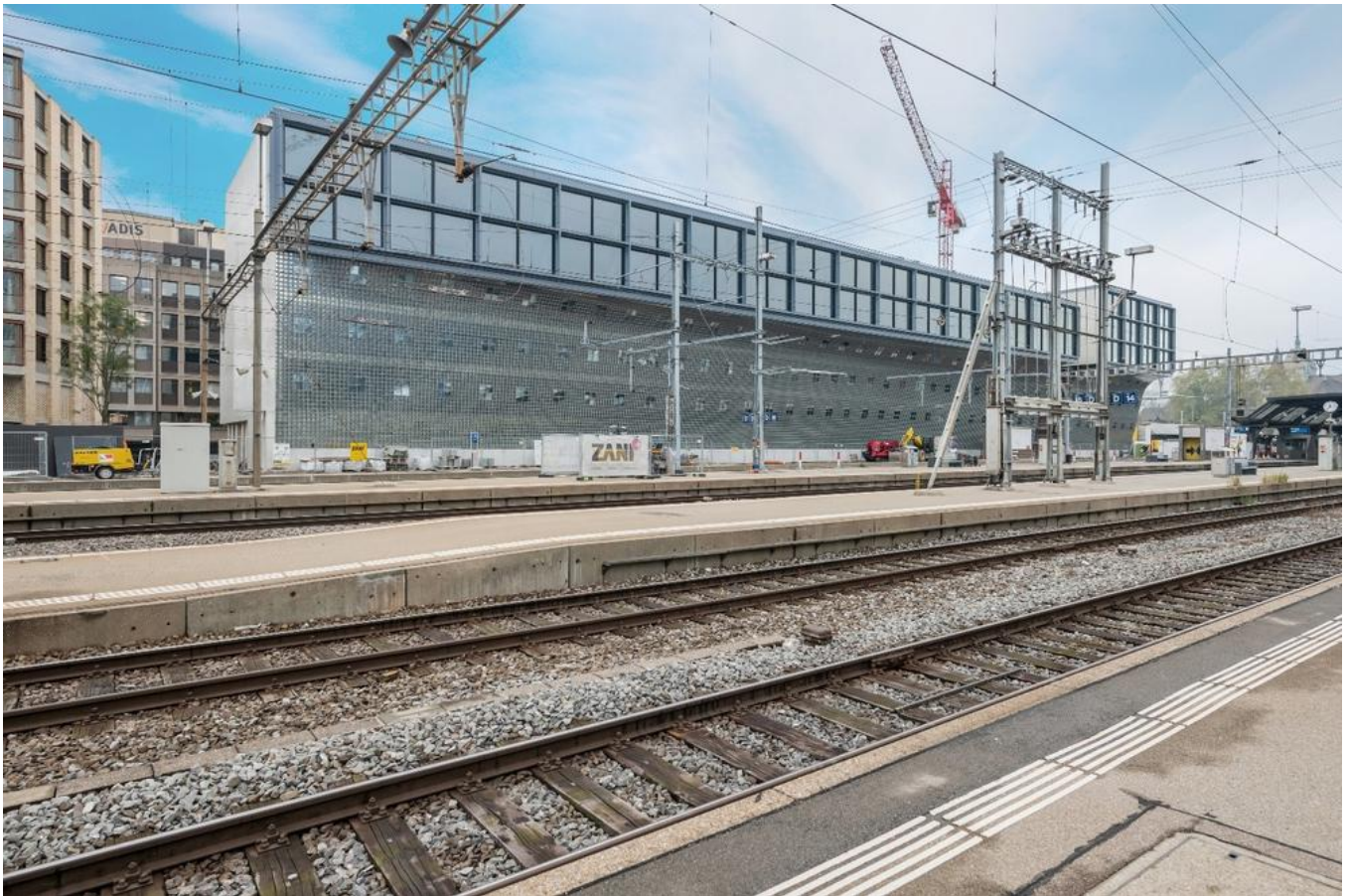
The eye-catching glass brick façade at the Zurich's central station, with its multiple curves, represents a technological milestone for PORR. Source: PORR
