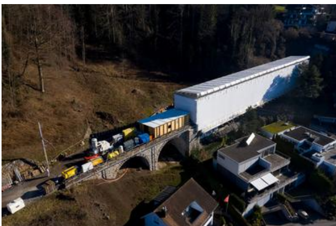
The steel bridges had to be encased for the corrosion protection work. Source: PORR
