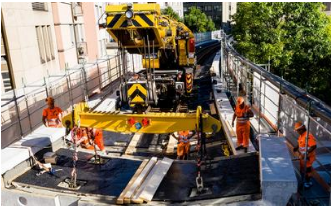
A new railbed with concrete elements was rerouted over an existing viaduct. Source: PORR
