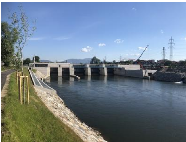
While work continues in the central reservoir channel (right), the weir and fish pass are already completed (left). Source: PORR
