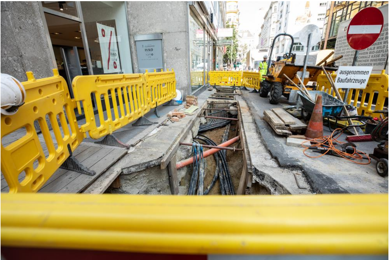
The cramped conditions around the construction area presented various challenges for the WIBEBA team. Source: PORR
