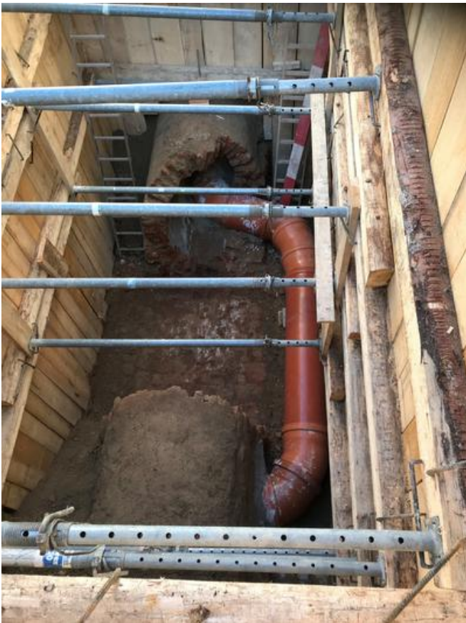
A specially built bypass ensured the sewage system continued to operate. Source: PORR
