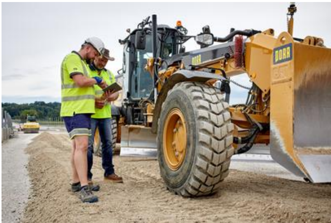
Numerous measures are being implemented in the Wieselburg bypass project to protect both people and planet. Source: PORR
