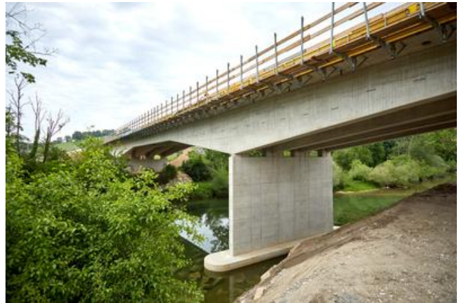
The consortium is building 14 of the 17 new bridges on the new route. As well as a number of smaller structures, these include the north and south bridges over the River Erlauf. Source: PORR
