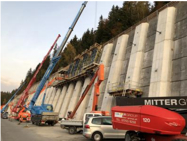
The pilaster strips on the anchor wall were concreted after the anchor holes had been drilled. Source: PORR Specialist civil engineering
