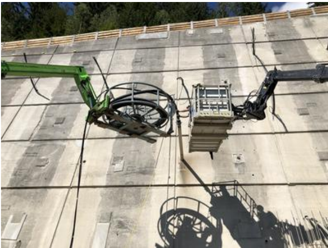
Altogether, 167 permanent strand anchors were installed on the Hochmais anchor wall, making 4,615m of anchors in total. Source: PORR Specialist civil engineering
