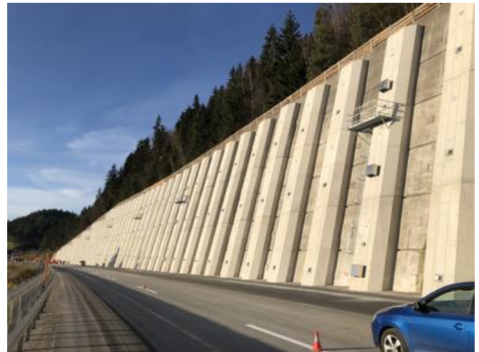
Regular monitoring of the anchor walls is facilitated by fifteen measurement cross-sections, fitted with 32 force plates and 25 extensometers. Source: PORR Specialist civil engineering
