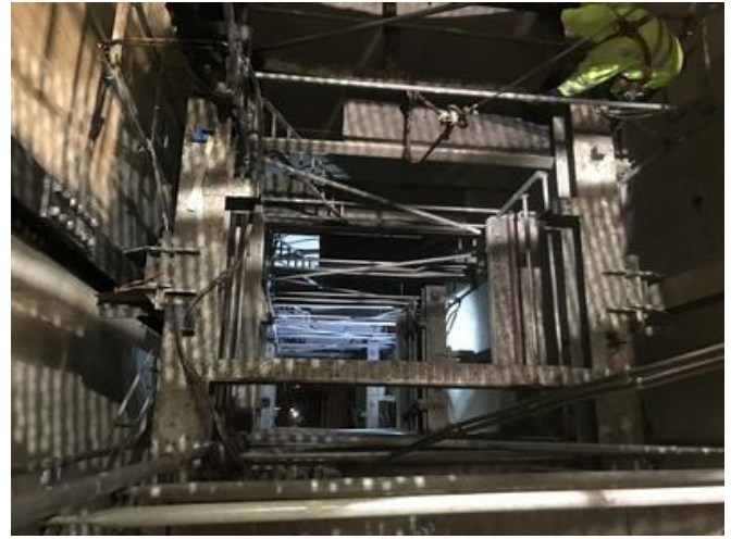
PORR built a 560 m 3 interior scaffold for safe removal of the steel parts. Source: PORR
