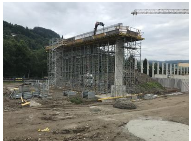
Due to their high dead load, the girders could not be delivered as pre-cast components, as specified in the tender, but had to be constructed in-situ instead. Source: PORR
