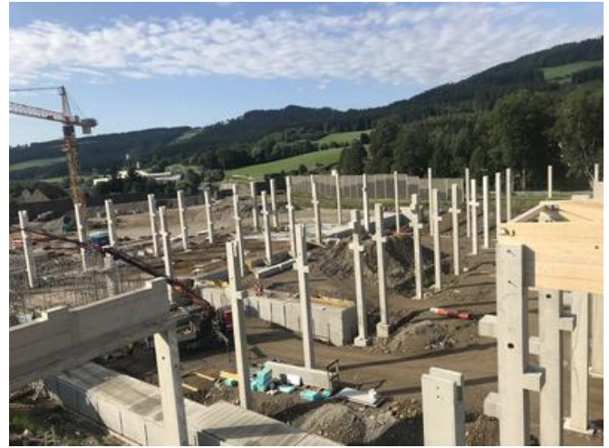
PORR carried out the surveying work for the 144 footings and columns itself. Source: PORR
