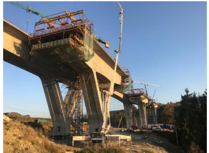
Sliding devices were used to concrete the individual bridge segments. Source: PORR
