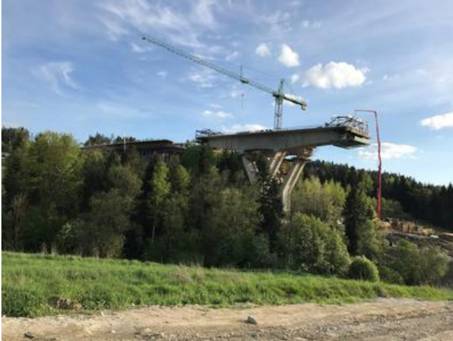
The bridge is about 50m high at its highest point. Source: PORR
