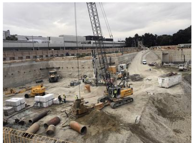
The deep wells for dewatering were made with large bore holes. Source: PORR
