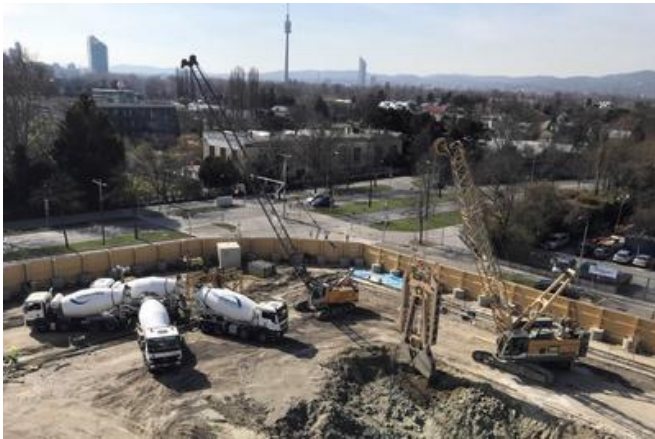
PORR was able to shorten the construction period considerably by separating the structural diaphragm wall from the jet-grouted groundwater sealing wall below it. Source: PORR
