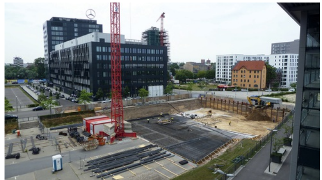
Development site in July 2014 shortly after start of structural work Image: PORR AG
