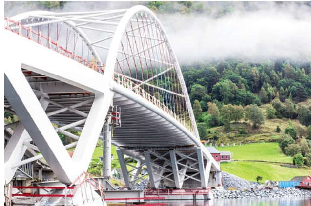
The final section of the Loftesnes Bridge was concreted in place in August. Image: PORR AG
