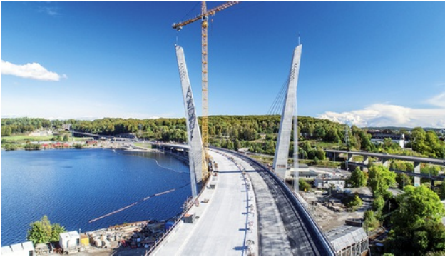
From the final section in July to the handover on 16 November – the PNC Norge team is connecting the inhabitants of Larvik via the Farris Bridge. Image: PORR AG
