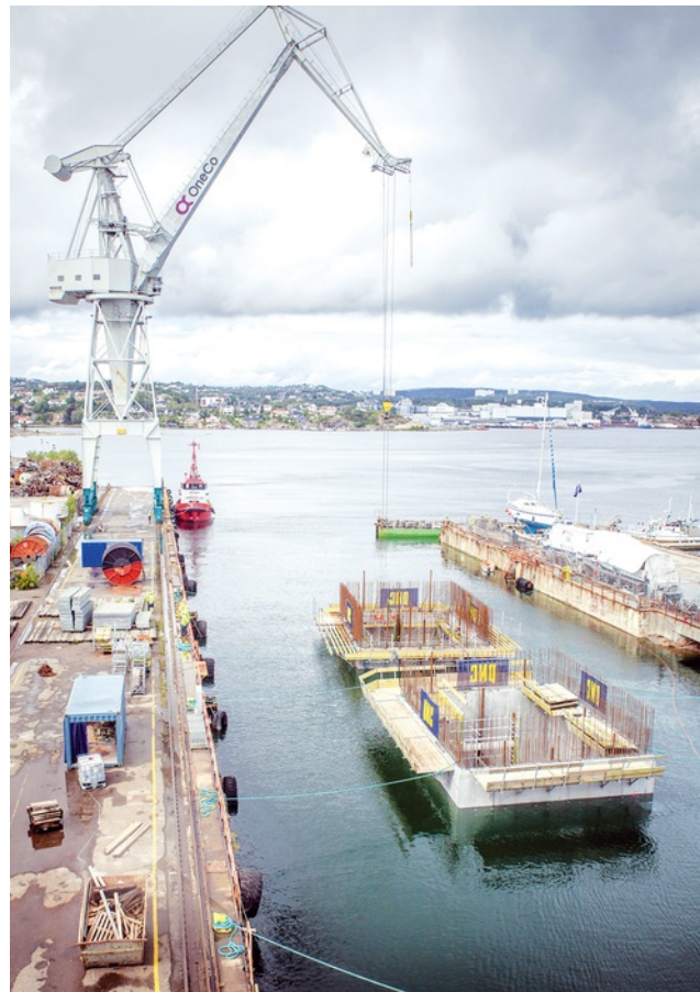
The flooding of the caissons for the Varrod Bridge proceeded smoothly. Image: PORR AG
