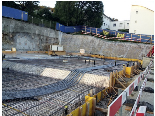
Geothermal probes in the floor panel Image: PORR AG
