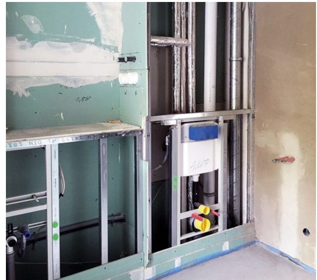
Service lines with inlet at floor level Image: PORR AG
